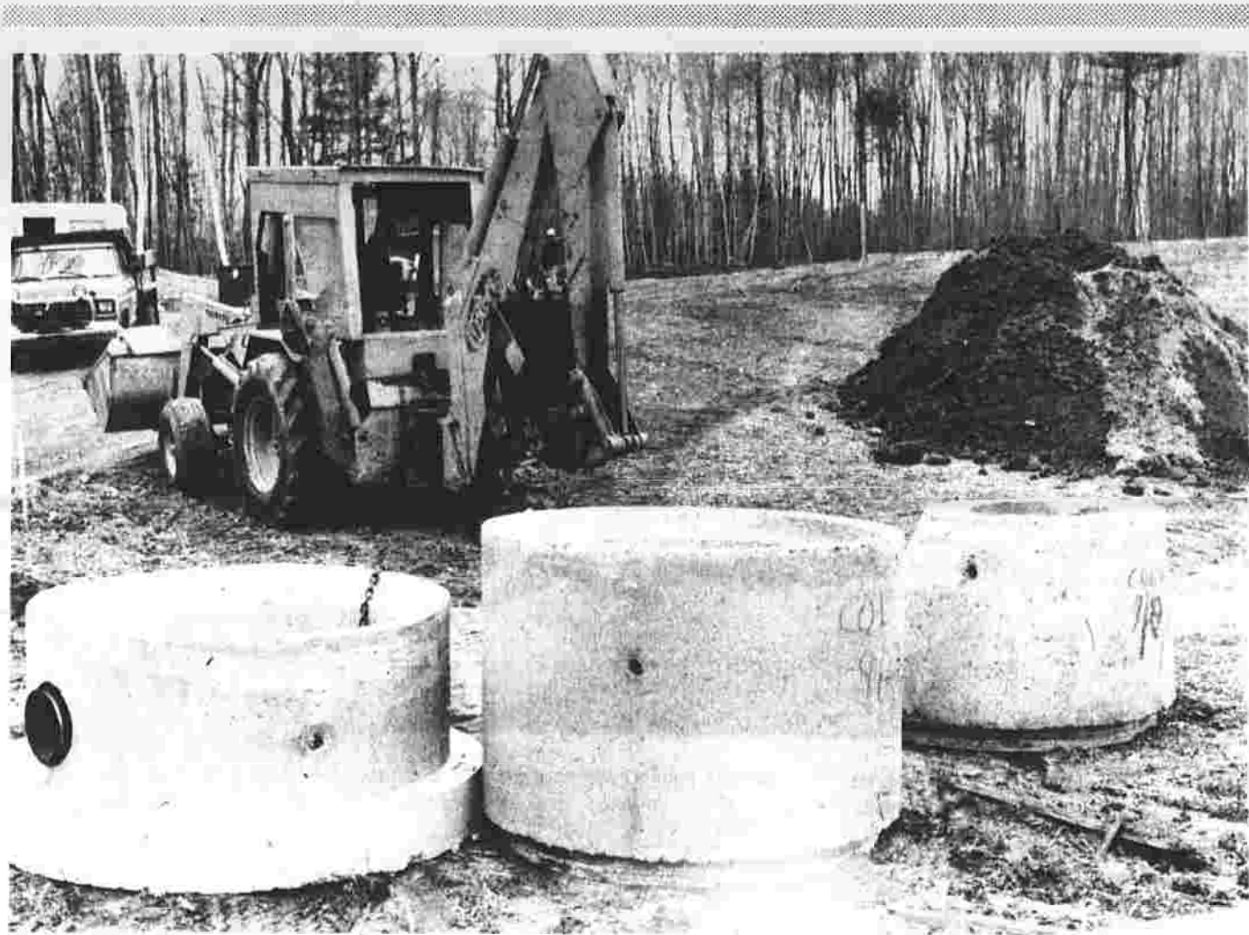
Work is progressing on several projects in the Buckland Industrial Park including a new building under construction for Tomko Electric. In the above photo, sections of drain pipes await replacement. (Herald photo by Pinto)
